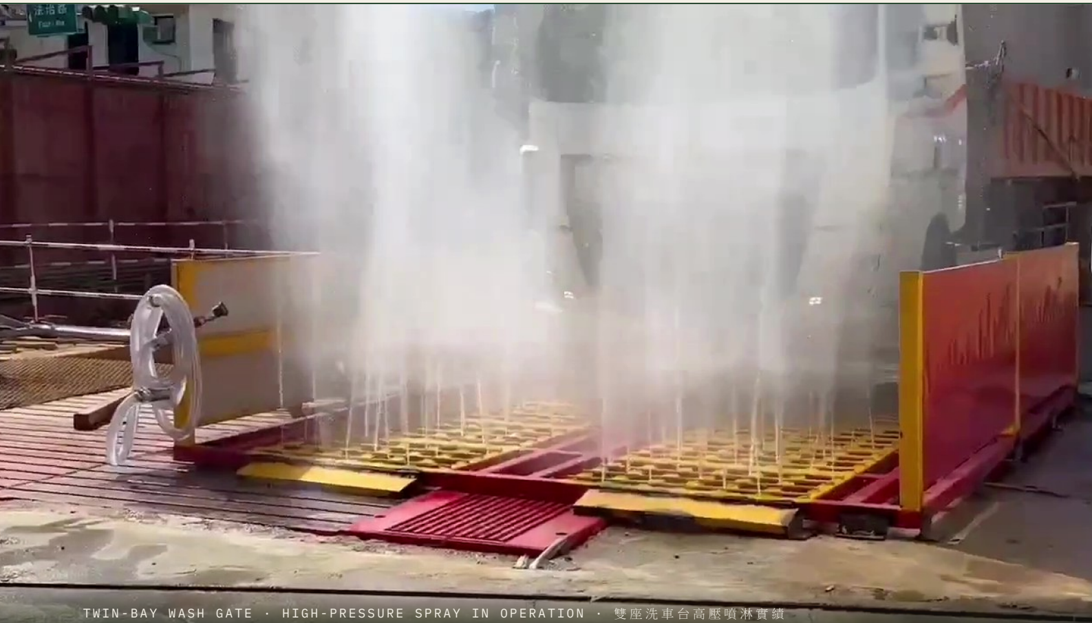
TWIN-BAY WASH GATE · HIGH-PRESSURE SPRAY IN OPERATION · 雙座洗車台高壓噴淋實績
